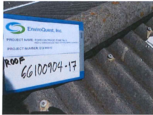
Photo #20: Roof ridge. Non-asbestos containing black sealant. Asbestos-containing cementitious roof ridge.
