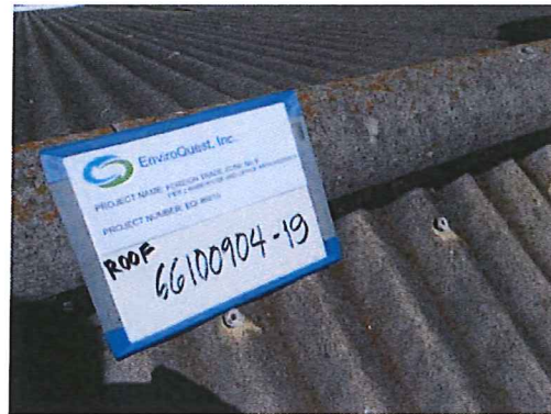
Photo #22: Roof ridge. Non-asbestos containing black sealant. Asbestos-containing cementitious roof panel.
