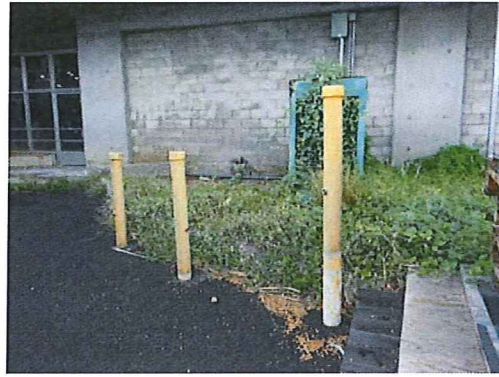
Photo #53: Lead-based painted yellow bollards.
