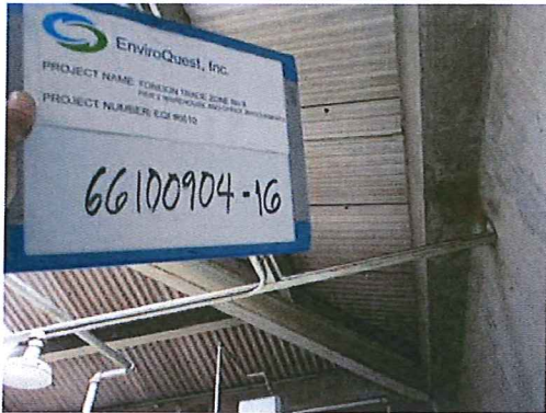
Photo #19: Asbestos-containing corrugated roof panel.
