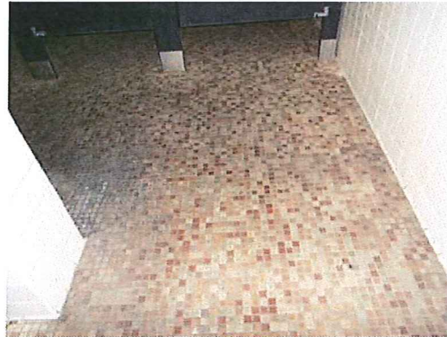
Photo #40: Ground floor, restroom. Non-lead based paint coated glazed tan ceramic floor tile.
