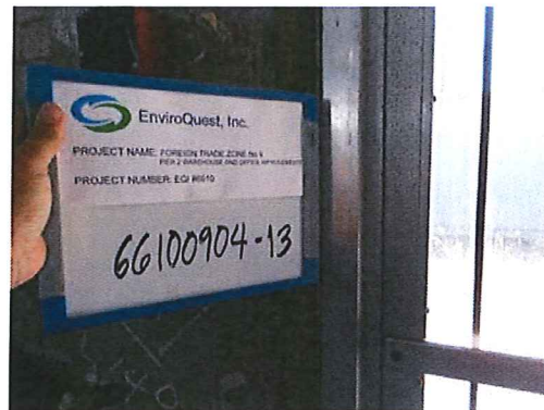
Photo #16: Ground floor, aluminum exit door frame. Asbestos-containing tan door caulking.
