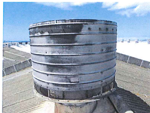
Photo #24: Roof exhaust fan. Asbestos-containing black felt coating under silver paint and black tar.
