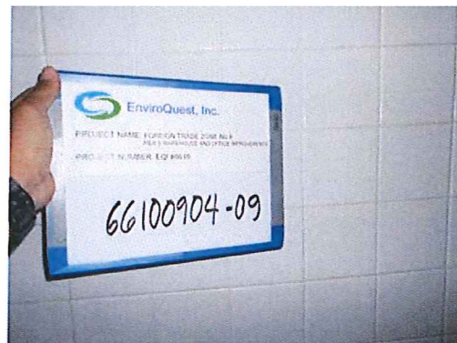
Photo #12: Ground floor, restroom. Non-asbestos containing white ceramic wall tile and grout.
