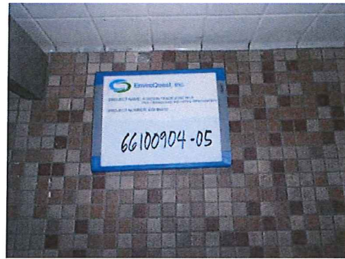
Photo #8: Ground floor, restroom. Non-asbestos containing tan ceramic floor tile and grout.
