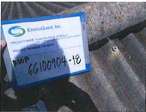
Photo #21: Roof ridge. Non-asbestos containing black sealant. Asbestos-containing cementitious roof panel.
