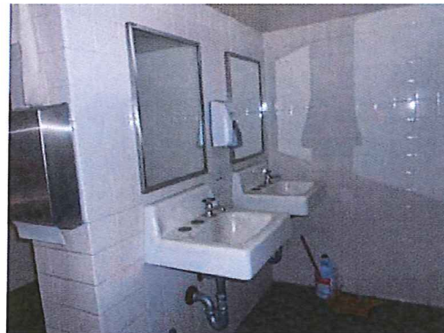
Photo #42: Ground floor. Lead-based paint coated glazed white ceramic wall tile.
