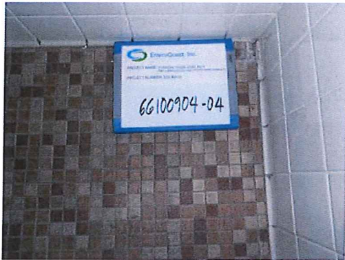
Photo #7: Ground floor, restroom. Non-asbestos containing tan ceramic floor tile and grout.
