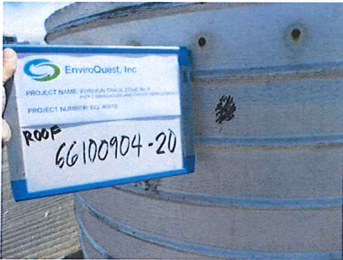
Photo #25: Roof exhaust fan. Asbestos-containing black felt coating under silver paint and black tar.
