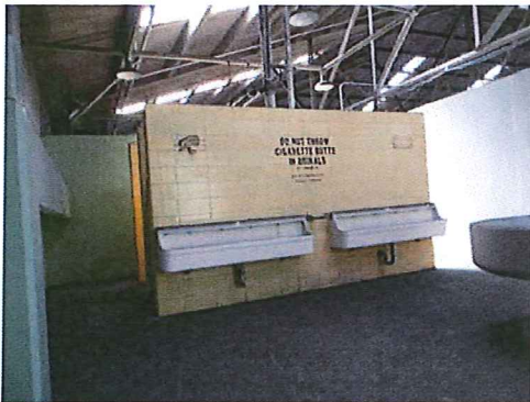
Photo #48: 2nd floor, urinal area. Non-lead based paint coated glazed beige ceramic wall tile.
