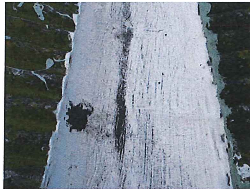
Photo #36: Roof gutter. Asbestos-containing roofing felt under non-asbestos containing elastomeric coating and tar.
