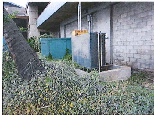
Photo #55: Non-lead based painted blue and blue-green transformer.
