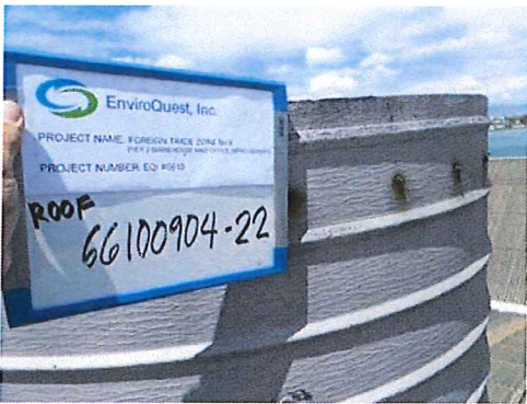
Photo #27: Roof exhaust fan. Asbestos-containing black felt coating under silver paint and black tar.
