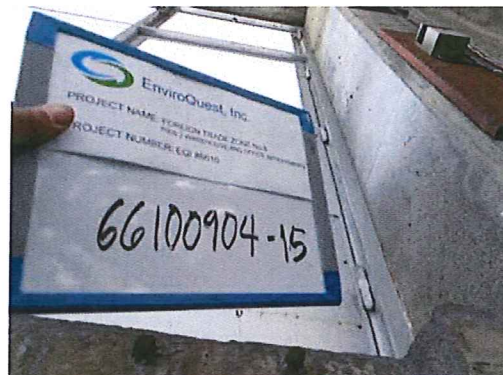
Photo #18: Aluminum window frame. Asbestos-containing tan window caulking.
