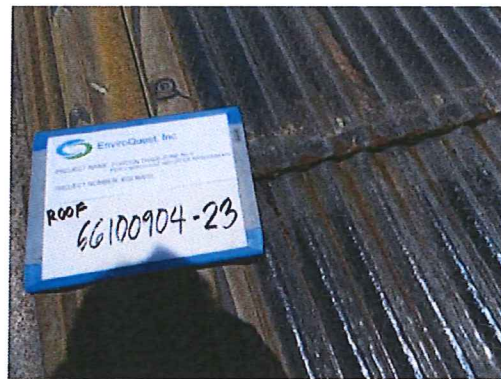
Photo #28: Roof skylight. Asbestos-containing debris from cementitious roof panel on the non-asbestos containing black sealant.
