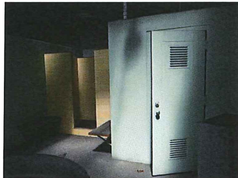
Photo #49: 2nd floor, storage room. Non-lead based painted green wall and door.
