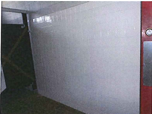
Photo #41: Ground floor. Lead-based paint coated glazed white ceramic wall tile.
